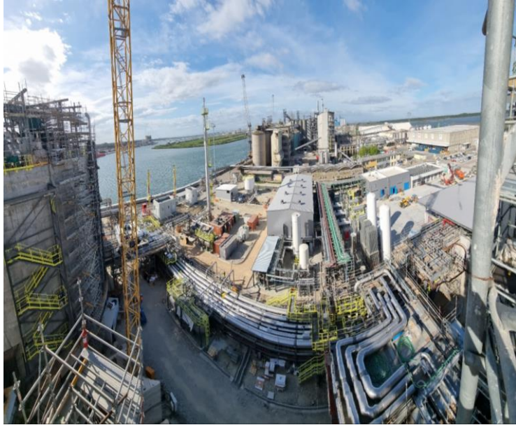
General view from the tanks
