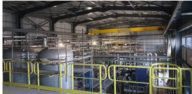
Internal Areal – re liquefaction
